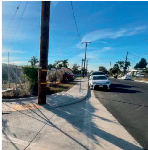
Top left photo: the project involved the relocation of about 30 utility poles that conflicted with the street widening and reconstruction.
